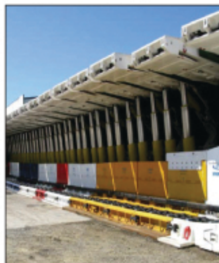
INBYE roof supports system at Carborough Downs Mine.
