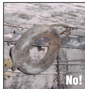
Cable Anchor Too Close to Feeder Cable
